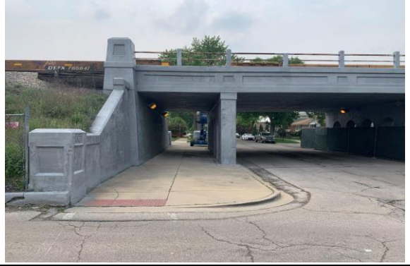
Chicago 66 th Street Viaduct, after Dan's Community Project
