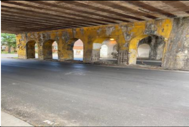
Chicago 63rd Street Viaduct with yellow lead based paint before Dan's Community Project
